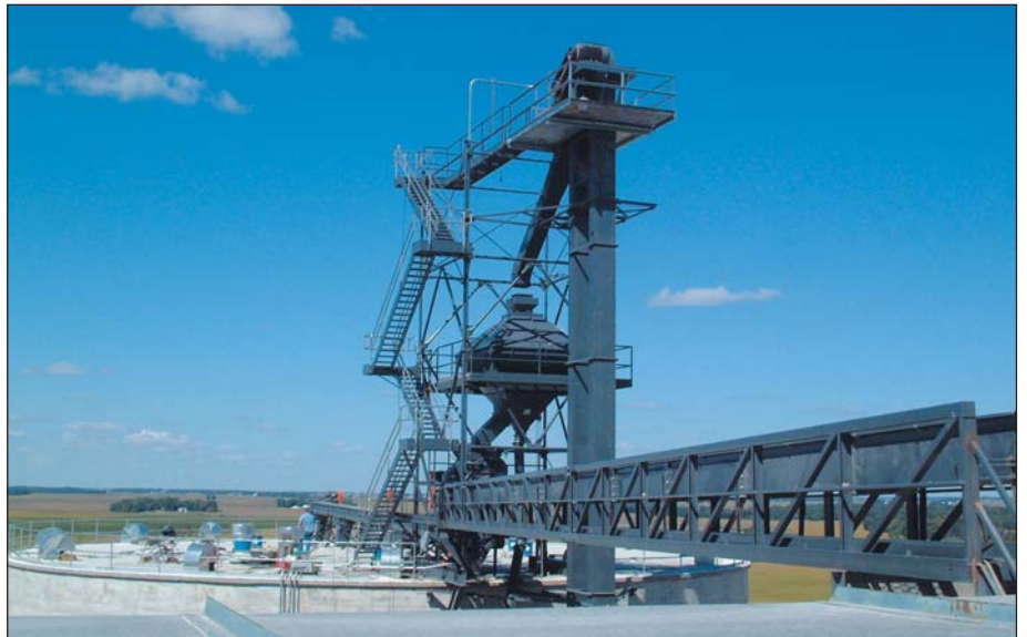
20,000-bph reversing drag conveyor runs from the elevator’s original concrete house out to the new tank. Also visible is a new 20,000-bph leg and 20,000-bph gravity cleaner. Photo courtesy of Hoffmann Inc.
