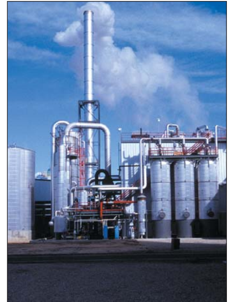
Distillation column is used to separate moisture from grain alcohol, producing a 190-proof product for further dewatering.
